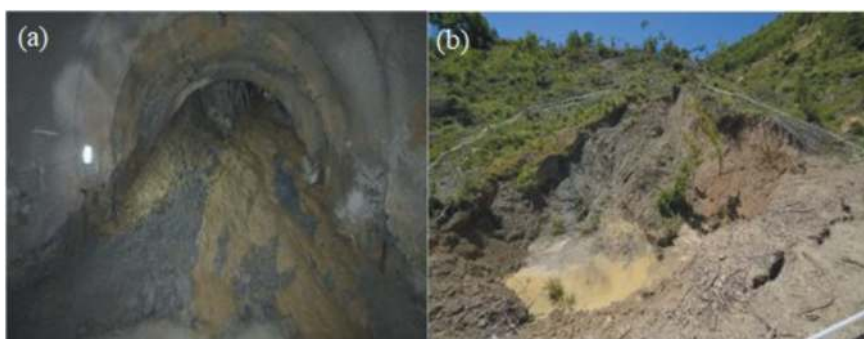
Figure 4. Photos of the chimney-shaped collapse at the tunnel entrance (Sta. 0+164): (a) Internal view showing the failure of the primary lining and accumulation of debris; (b) External manifestation of the collapse on the natural slope surface, illustrating the upward propagation of the instability.
