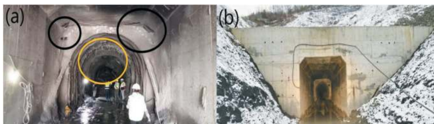
Figure 5. Observed structural distress and the remedial measure: (a) Severe deformation of the primary lining with highlighted areas of crown distress and longitudinal cracking; (b) View of the stabilized structure following the 20 m extension of the conduit.
