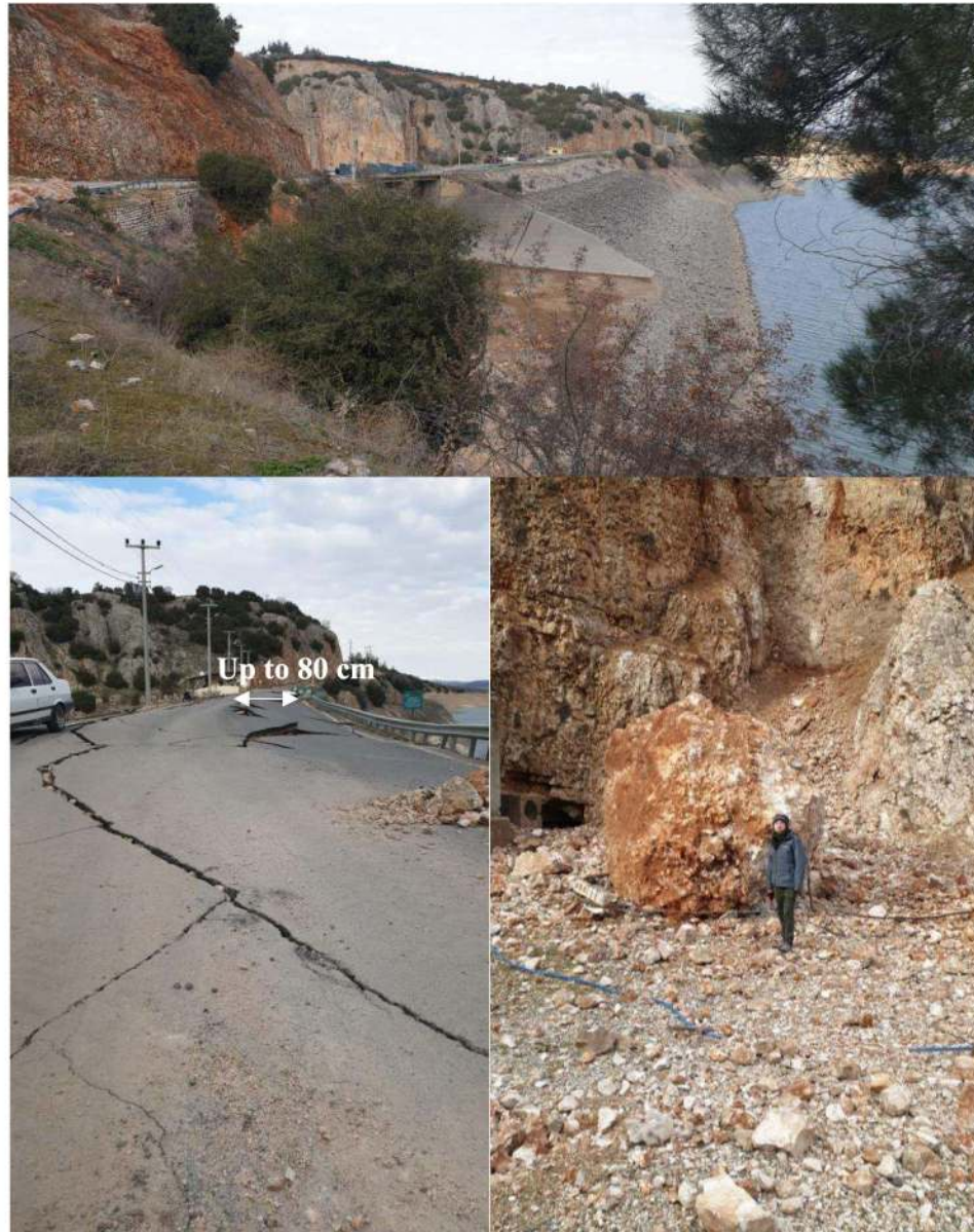
Figure 3: Photographs taken during post-earthquake inspections of Kartalkaya Dam, illustrating moderate to major levels of cracking along the crest.
