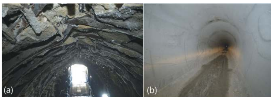
Figure 6. View of the tunnel sections: (a) Close-up view of the structural collapse, showing twisted steel ribs and fractured shotcrete resulting from excessive ground pressure; (b) View of the final completed concrete lining, showing the stable condition achieved after overcoming the initial support failure.
