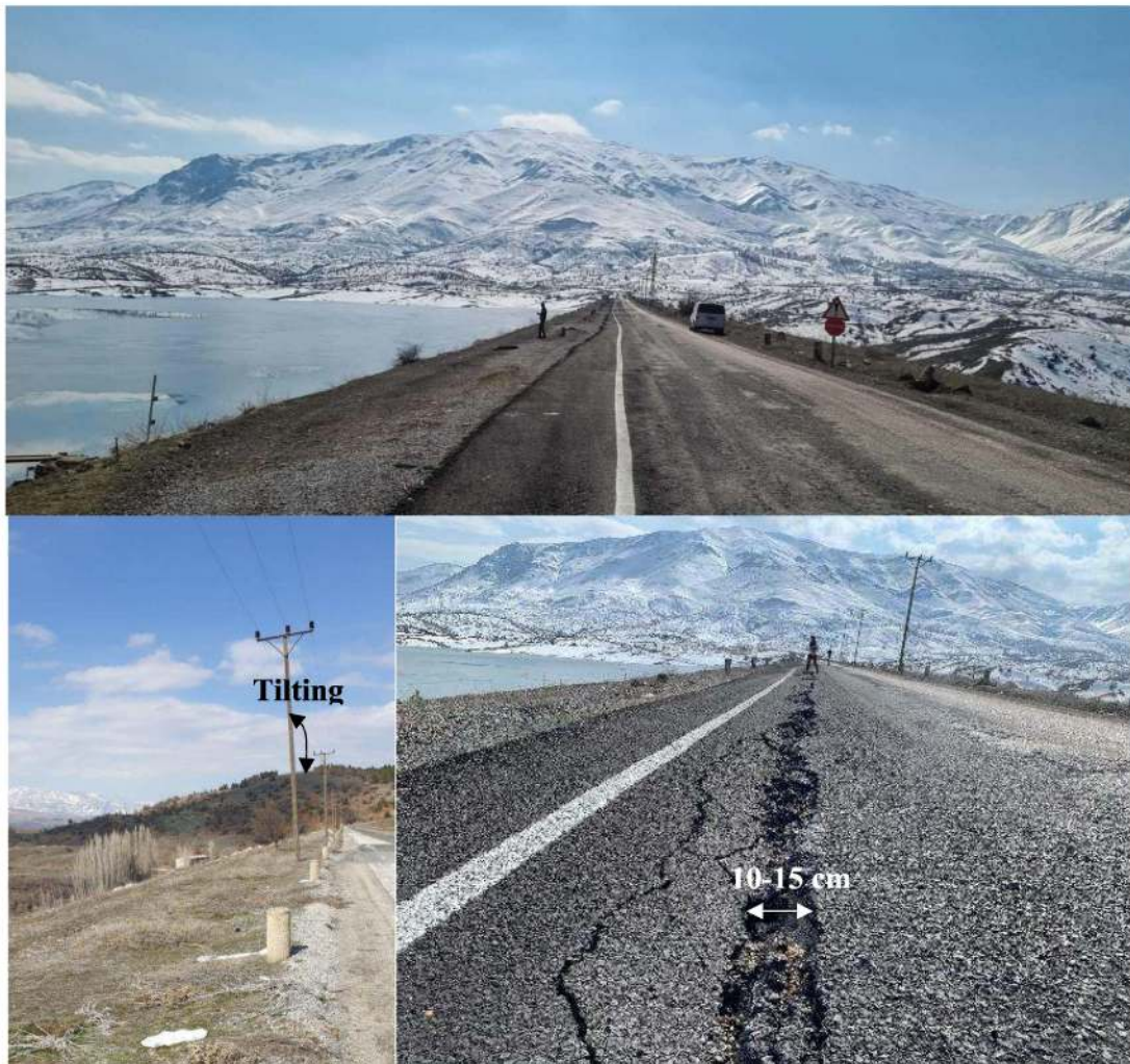
Figure 2: Photographs taken during post-earthquake inspections of Sürgü Dam, illustrating moderate levels of cracking along the crest.
