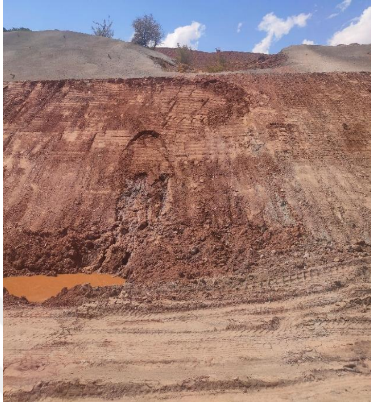
Figure 4.81. Front view of the excavation slope before the main failure
